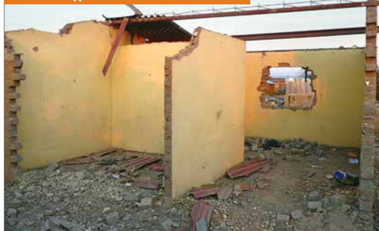
Photograph 2: Collapsed wall panel due to un-bonded central wall support
