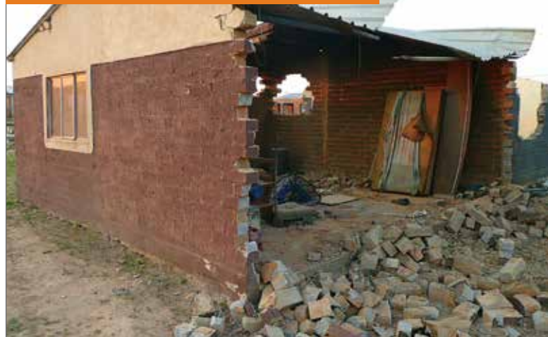
Photograph 1: Collapsed wall panel due to tooothing-in of masonry units at return walls
